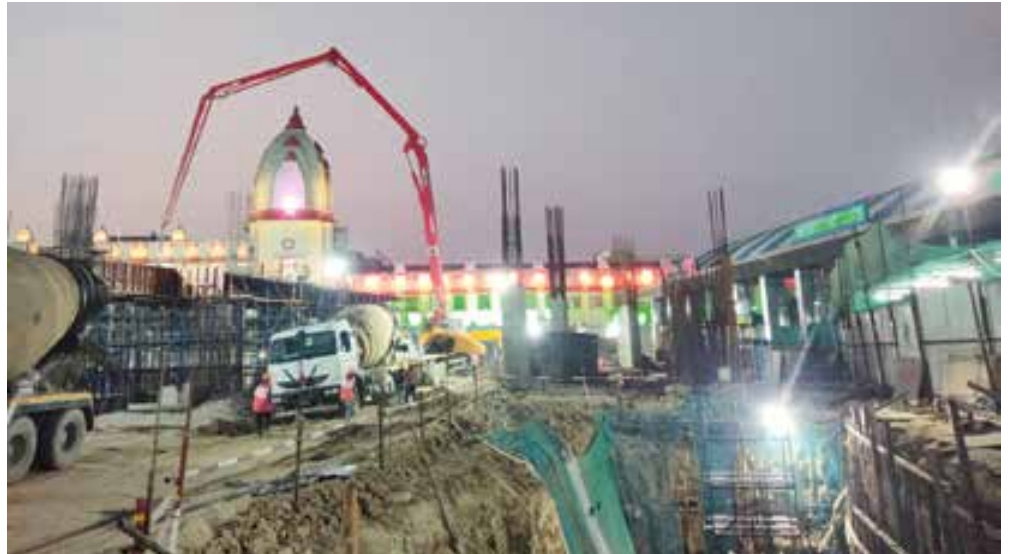
Big plans in India: The cable car Varanasi 1 is currently under construction – with five stations, a length of 3.76 kilometers, and a capacity of 3,000 persons per hour. Varanasi 2 (green line) is scheduled to be tendered later this year. © SALZMANN
